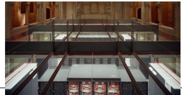
MARENOSTRUM (BSC, SP) IBM System x iDataPlex system– 48,448 cores
